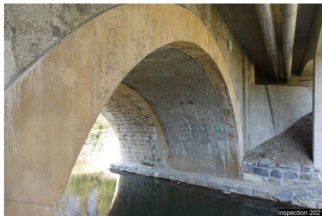
Pd1 Pedestal 301 Wetlands Internal face. Slight cracking of the visible surface with old limestone.
