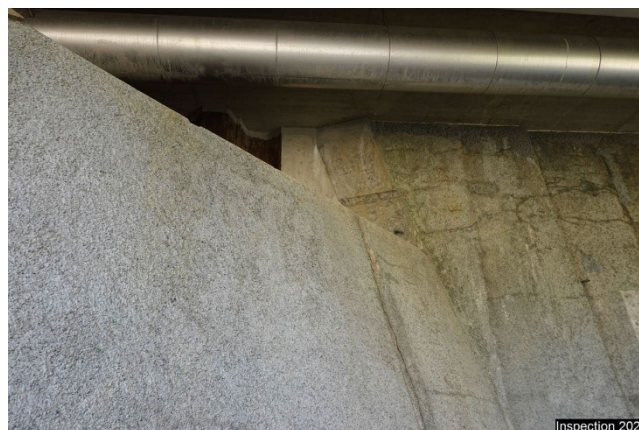
CuDr0 Right wing wall axis 0 1209 Joint cracks Vertical joint. Crack in plaster mortar.
