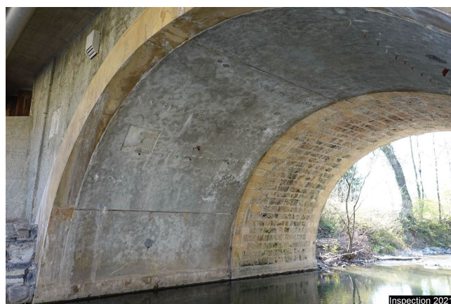
VoDr Voûte Droite 301 Wetlands Distributed over the entire element. Slight surface cracking visible with old calcareous deposits.
