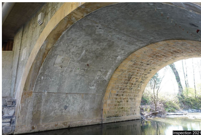
Pd0 Pedestal 1210 Longitudinal cracks Internal face. Slight cracking of the visible surface with old limestone.
