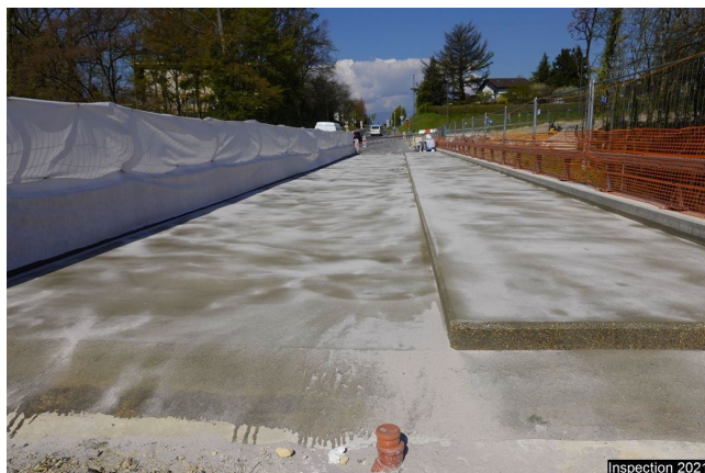
Re Coating \ other findings On entire deck. Coating not yet installed at time of inspection.
