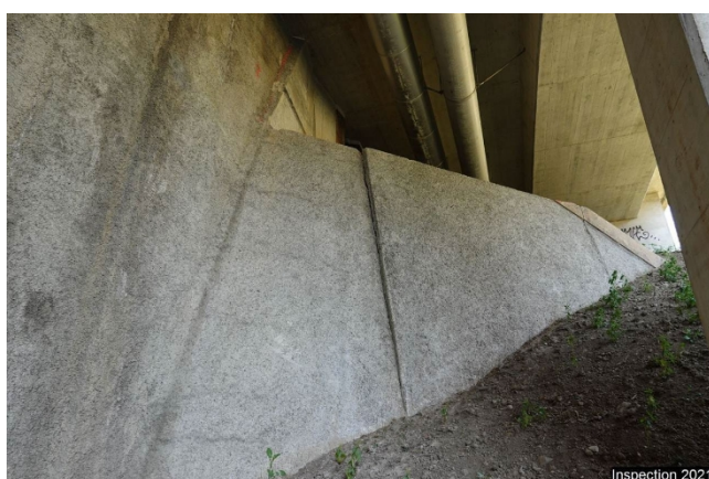
CuDr1 Right wing wall axis 1 1209 Joint cracks Vertical joint. Crack in plaster mortar.
